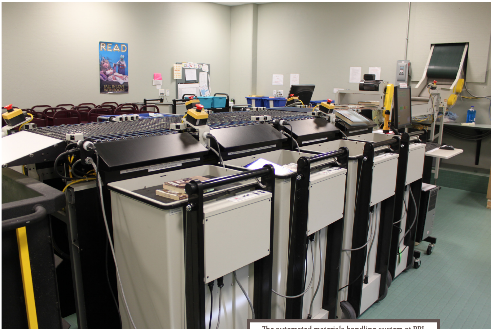
The automated materials handling system at PPL
